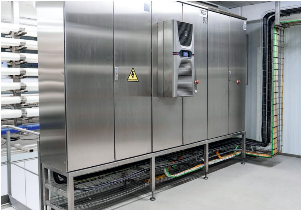
Liquats Vegetals also uses Rittal cooling units.
