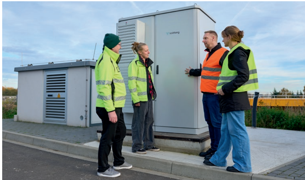
Installed on its own foundations at AWA, the Voltfang storage system does its job with absolute reliability.
